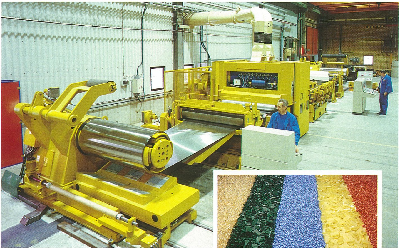
A new surface-treatment line for wide steel belts has been installed at the facilities in Sandviken.
