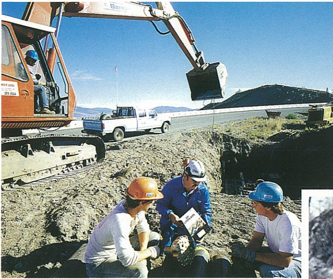
Canada. Claes Wikström takes part in drilling a hole for a cable under a motorway in British Columbia.
