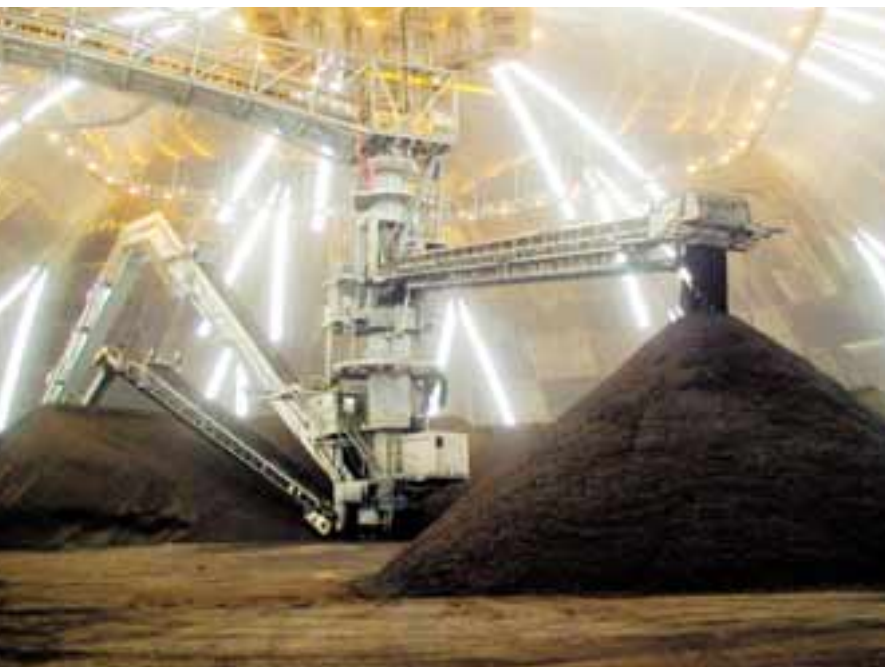
The business area's materials-handling systems play a key role for customers involved in mines, quarries, power plants, harbors and terminals.
